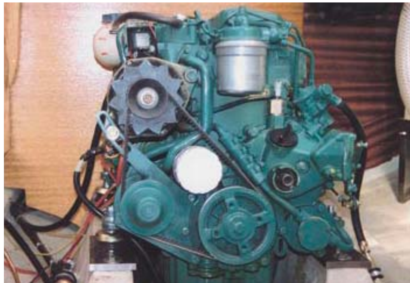
Example of RAB installation on a 3 cylinder diesel engine power pack.
